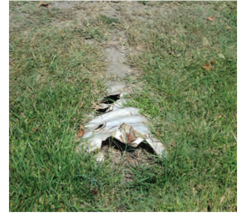
Clogged drain pipe under Park Road
