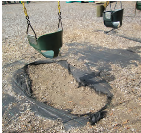
Safety surfacing not in compliance
