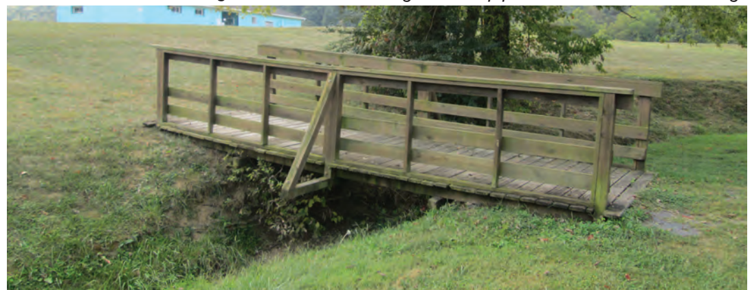
Stream banks eroding at pedestrian bridge location
