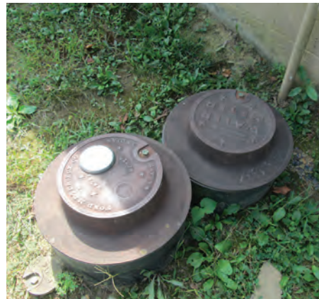
Water meter at restroom facilities
