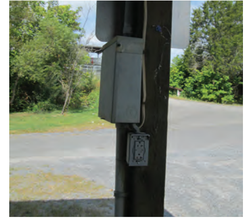
Electric at the First Bank Park Shelter
