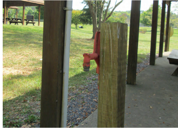
Water connection at the Kiwanis Park Shelter
